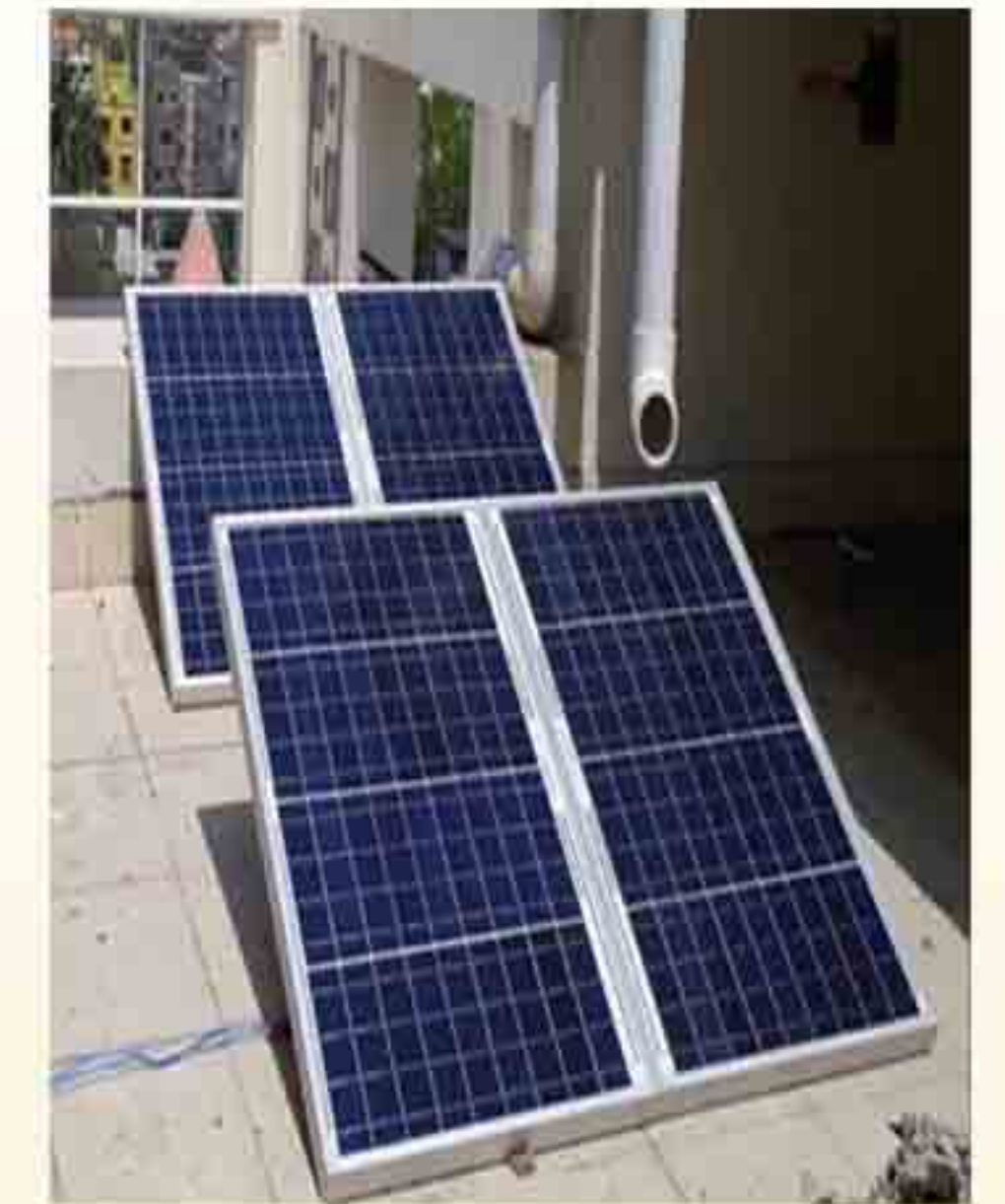
Rooftop Solar Plant
