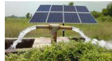
Solar Water Pumping System
